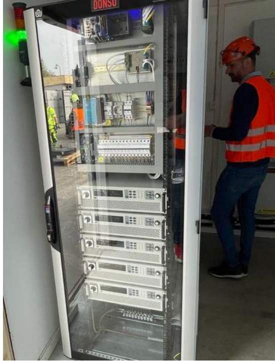
Figure 4 – Donsö central cabinet
