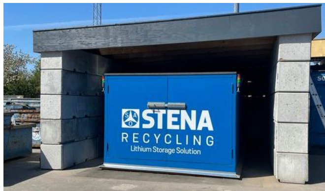
Figure 1- Stena Recycling Battery Center in Farum Denmark
