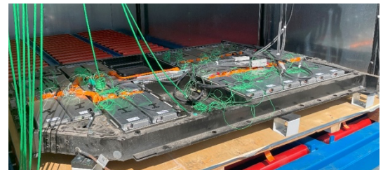
Figure 2 - EV battery pack prepared for discharge
