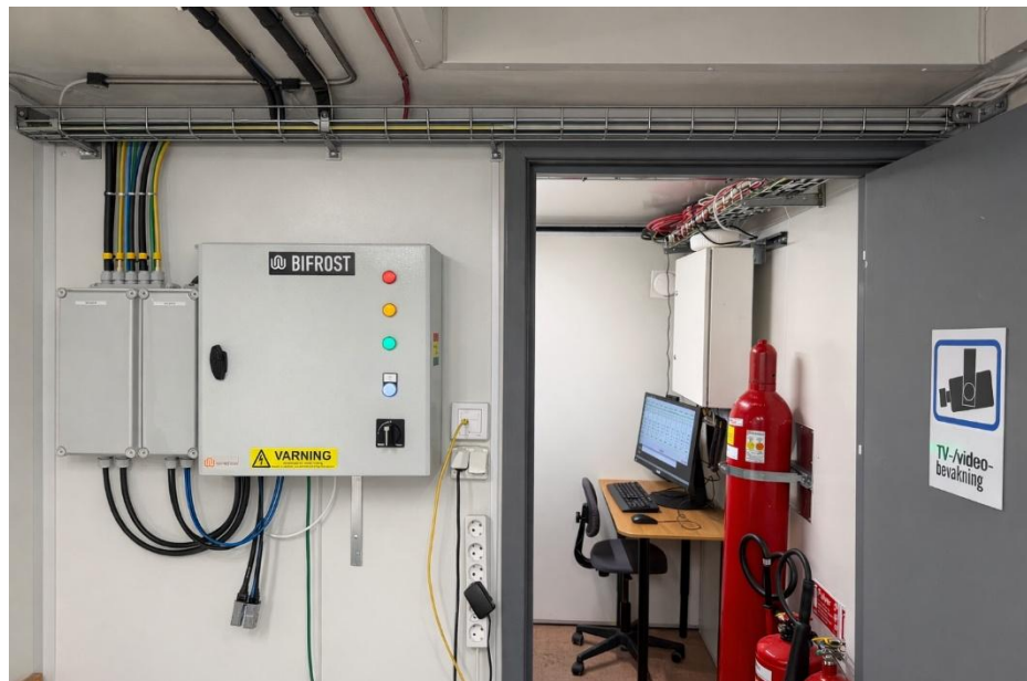
Figure 2 - WF Bifrost Connection Node and operator PC
